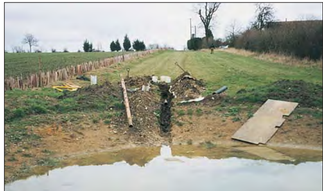
An agricultural field drain is intercepted and brought to the pond edge with pipework as a water supply
