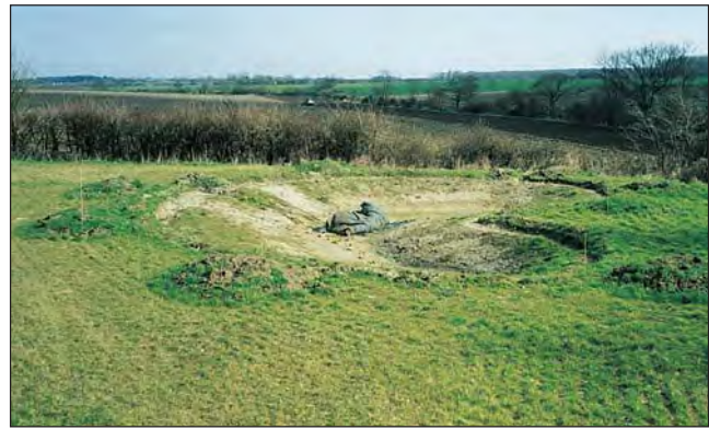
Lining a small (40m 2 ) pond on made-up ground. The pond has been dug and protective matting (centre) is unrolled to protect the underside of the heavy-duty butyl liner from below
