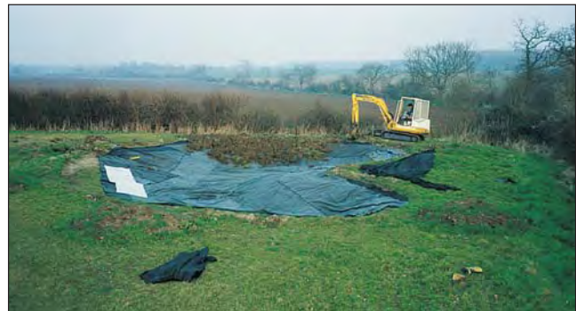
The butyl is put in place, and a further layer of protective matting (polyester) is placed on top. Topsoil is then spread over the pond base to a depth of 50-100mm
